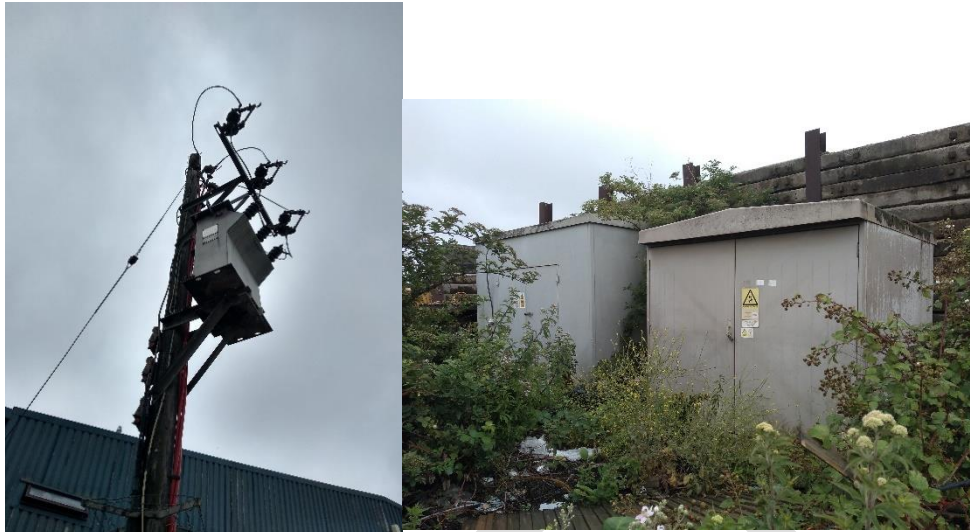
Figure 20: Some of the various transformers along the North Quay Road
