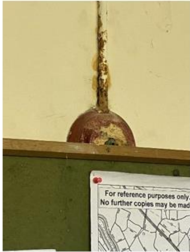
Office 5 – Corrode historic fire alarm
