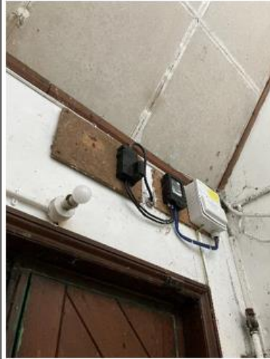
Office 6 – Electrical Distribution
