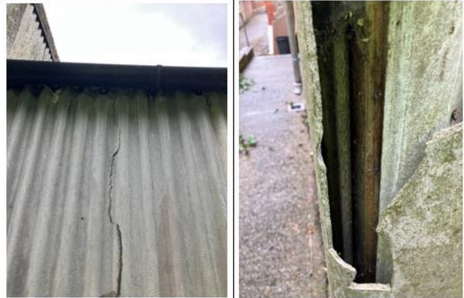
West Elevation 3- Crack in Fibre Cement Panel
