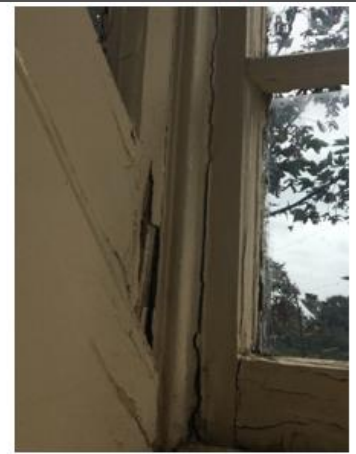
First Floor 8 – Wet Rot to Frames
