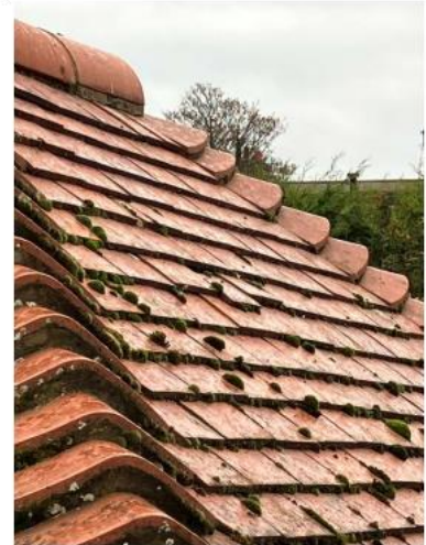
Roof 3- Broken tile
