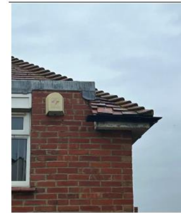
West Elevation 3 - Slipped roof tile
