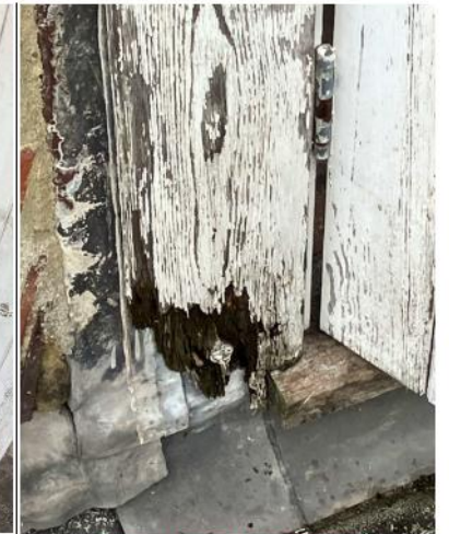
Roof 6 – Close up of door frame wet rot
