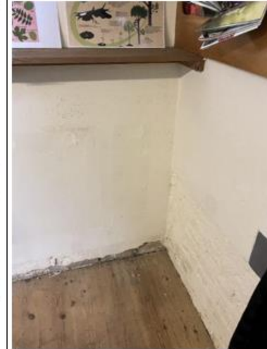
Office 4 – Flaking Floor Finish and Rising Damp
