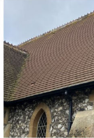
East Elevation 2 - Slipped Roof Tiles
