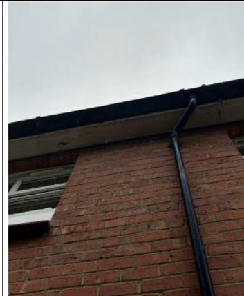
South Elevation 2 - Paint failure on soffits
