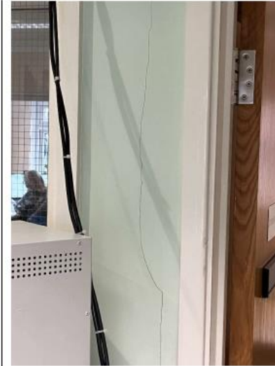
First Floor 13 – Hairline crack
