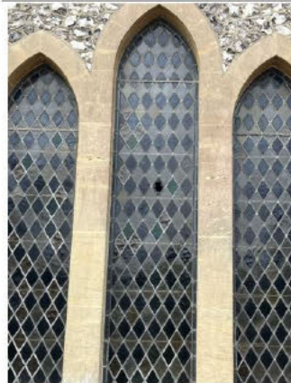
East Elevation 3 - Broken Glazing Section
