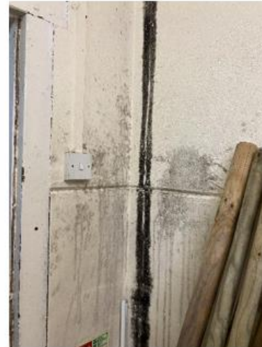
Morgue 6 – Stained Wall Finishes
