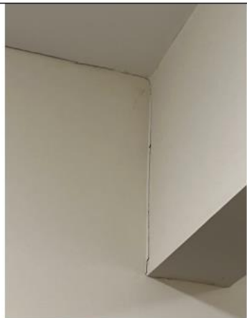
Second Floor 6 – Hairline crack
