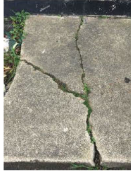
North Elevation 2 - Cracking to concrete step
