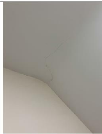
Second Floor 7 – Hairline crack to ceiling
