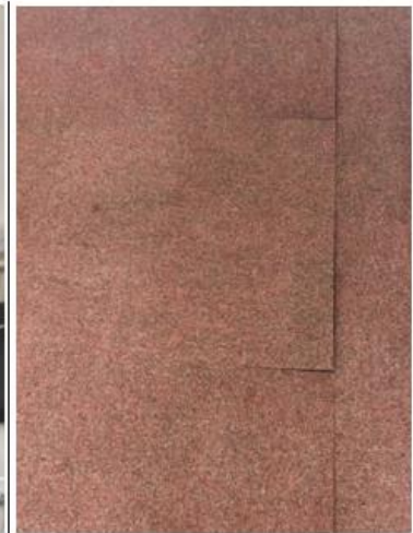
First Floor 6 – Carpet Lifting
