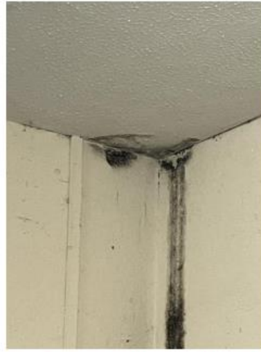
Morgue 5 – Stained Wall Finishes with Evidence of Moisture Ingress
