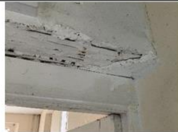
Morgue 7 – Damaged Wall Finishes, Requires Further Investigation
