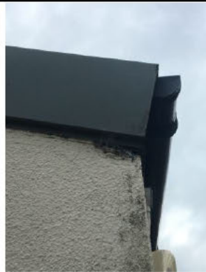
Fascias/Sofitts 2- Absent fixings to the fascias
