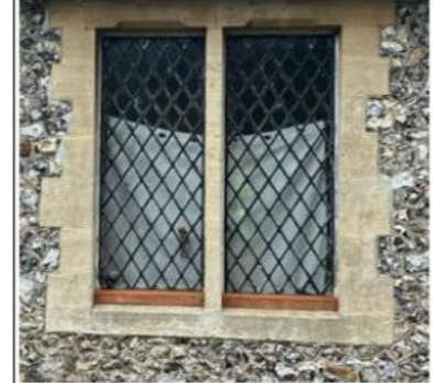
West Elevation 2 - Damaged Glazing Panes
