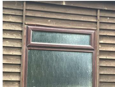
South Elevation 3- Broken Mastic Seal
