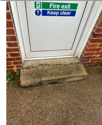
South Elevation 3 - Cracked concrete step
