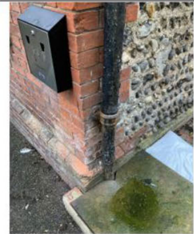
North Elevation 2 - Stone Slab and Failed Decorative Finish to Downpipes
