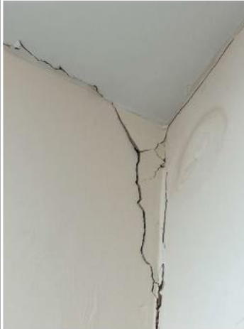
Second Floor 5 - Crack to wall and water stain between landing and meeting room
