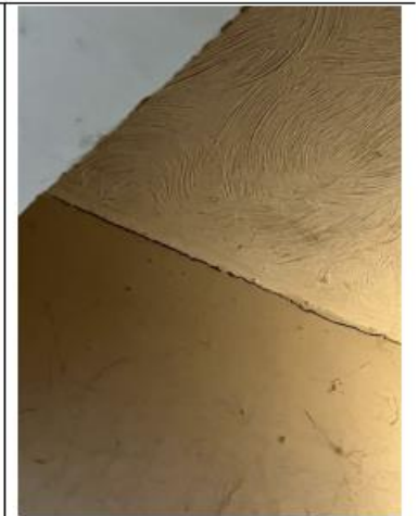
Storage Cupboard 2 - Cracked Wall/ Rendered Ceiling
