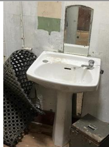
Sanitary Area 4 – Wash hand basin
