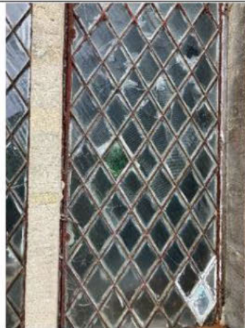
South Elevation 3 - Leaded Windows in Poor Condition
