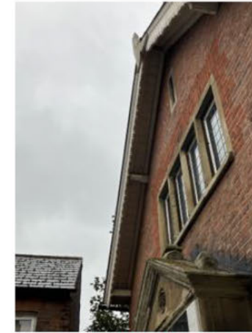
North Elevation 8 - Failed Paint to Soffits
