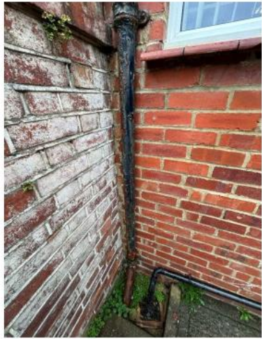
West Elevation 5 – Paint failed on downpipe and efflorescence on wall
