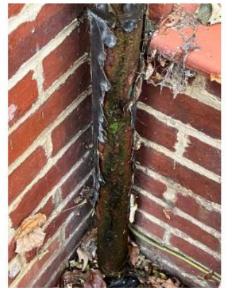
East Elevation 3 - Paint failure to cast iron downpipe
