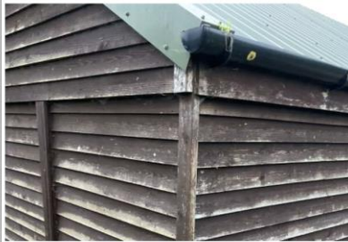
North Elevation 2- Blocked Guttering
