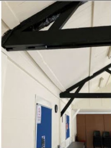
Hall 2 – Missing Knee Brace
