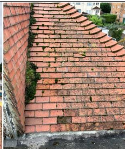
Roof 2- Moss and vegetation growth
