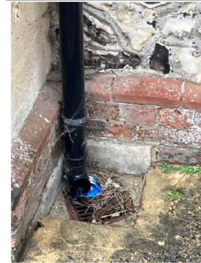
South Elevation 3 - Debris to Drainage Gully
