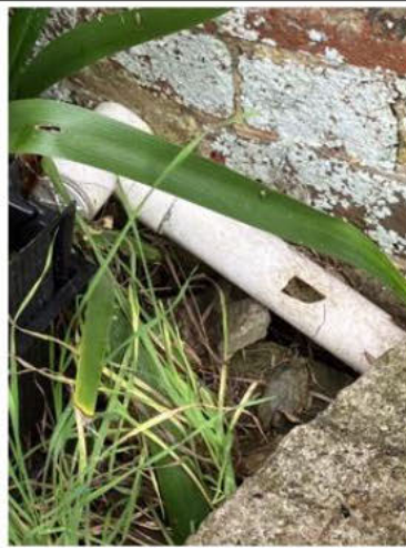
South Elevation 2 - Damaged Waste Pipe
