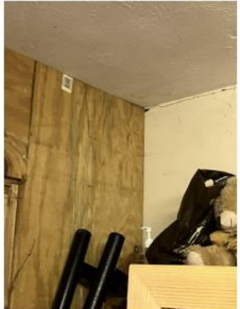
Storage Area 3 - Cracked Wall
