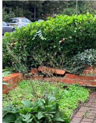
East Elevation 4 - Loose bricks from garden wall
