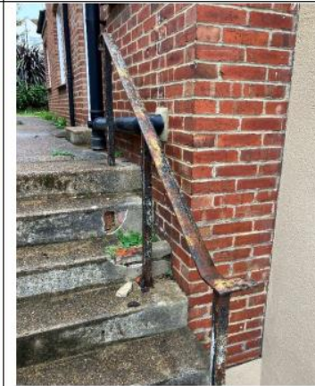
South Elevation 4 - Cracked cement on staircase
